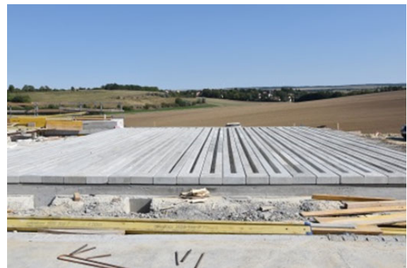
Fig. 1: Construction of the pilot on the Austrian motorway in 2017 by the Austrian motorway operator ASFINAG: A5, Satzengrabenbrücke Click here to watch the video
